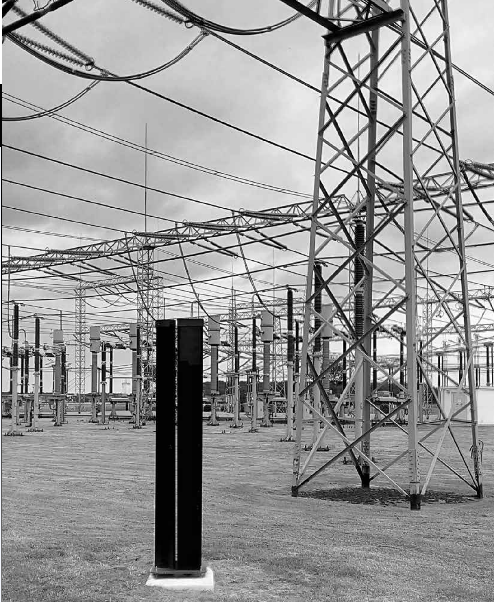
Dual Tech Barrier at German Power substation
